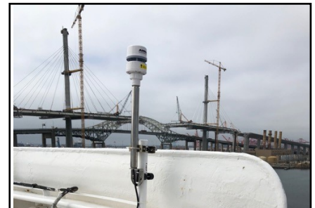
Installed weather station
