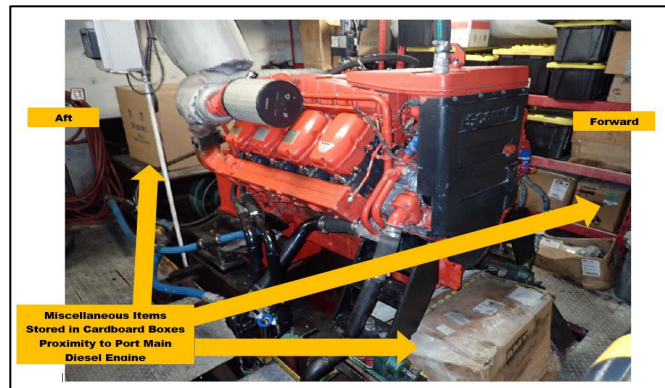
Figure 4: Combustible materials stored in the engine room.
